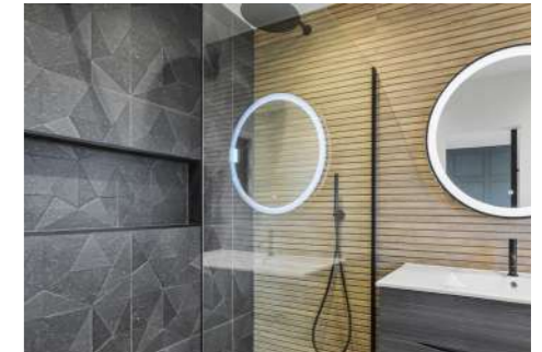
Bathroom & ensuite installations
